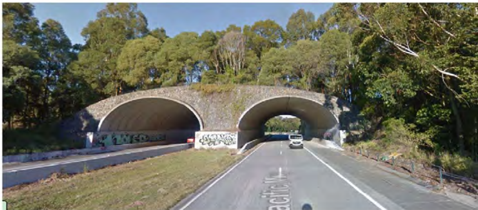
Figure 1. Dedicated fauna overpass across the Pacific Motorway in northern NSW. Once established, koalas (and other wildlife) are known to make regular use of such structures.
