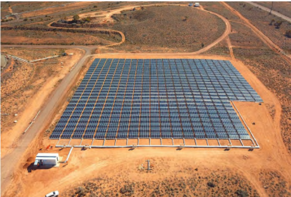
Figure 2-17. Example of a pre-fabricated (Maverick units) solar array, Port Bonython, SA (Source: 5B, 2020).
