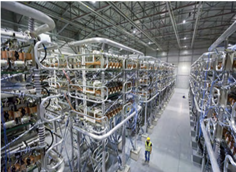
Figure 2-31. Internal view of a Voltage Source Converter (Source ABB Power Grids Pty Limited)
