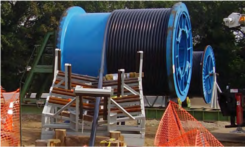
Figure 2-38. Photo example of motorised stand and roller placement used to install onshore cables (Source: Prysmian)
