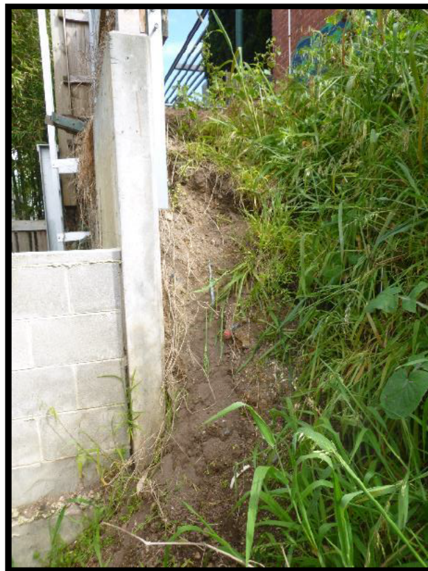
Photograph 10 – Photograph captured 13 October 2021. View of the western end of the subject land, looking west, at the north-east corner of 1 Campbell Grove (north-east corner of 1A Campbell Grove). Erosion of ground adjacent to retaining wall evident compared to November 2020 (photographs 7 – 9).
