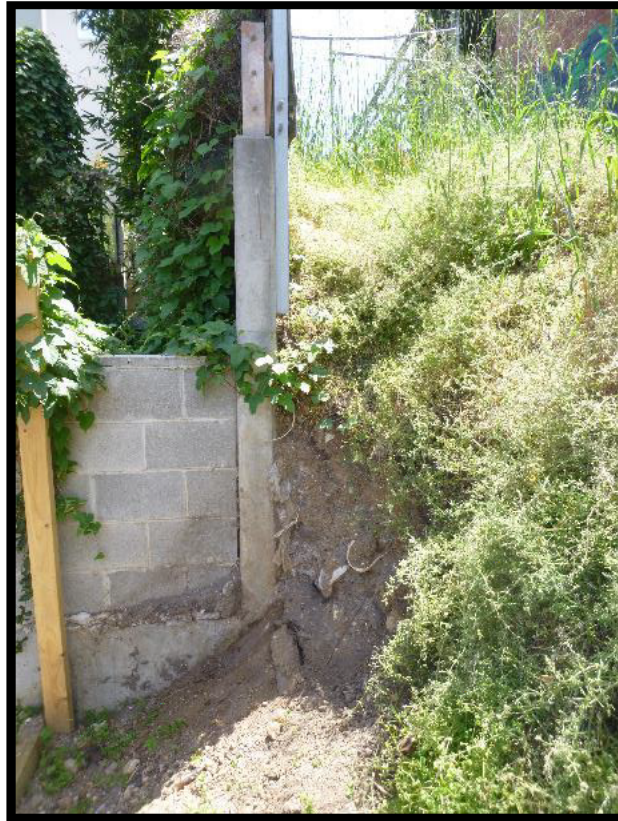
Photograph 7 – Photograph captured 19 November 2020. View of the western end of the subject land, looking west, at the north-east corner of 1 Campbell Grove (north-east corner of 1A Campbell Grove). Note vertical face of earth adjacent to concrete retaining wall.
