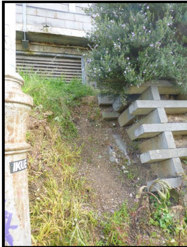
Photograph 6 – Photograph captured 14 October 2021. View of the eastern end of the subject land, looking north. Note localised erosion of land resulting in steep slope adjacent to crib wall.
