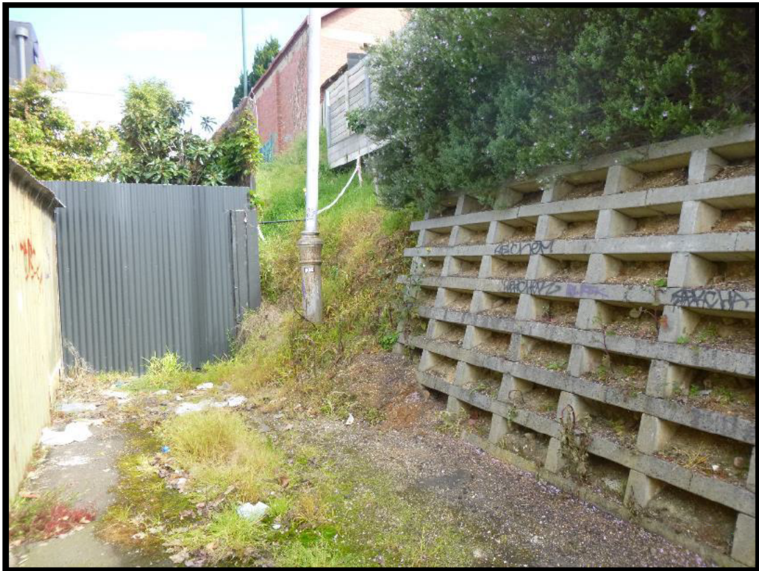
Photograph 4 – Photograph captured 13 October 2021. View of eastern end of subject land, looking north. Note spoil / loose material in laneway at the bottom of the batter, with vegetation growth over.
