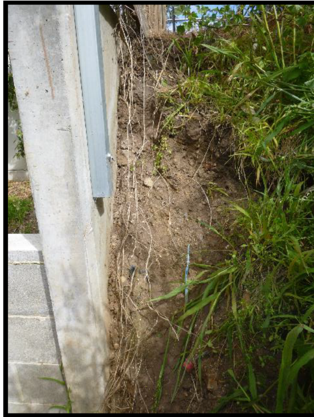
Photograph 11 – Photograph captured 13 October 2021. View of the western end of the subject land, looking west, at the north-east corner of 1 Campbell Grove (north-east corner of 1A Campbell Grove). Erosion of ground adjacent to retaining wall evident compared to November 2020 (photographs 7 – 9).
