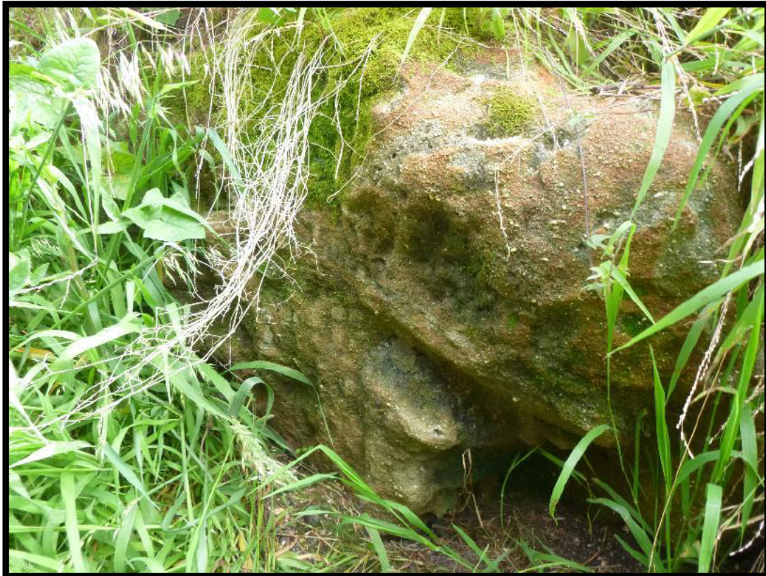
Photograph 17 – Photograph captured 13 October 2021. View of rock outcrop along the southern side of the subject land (i.e. long 1 Campbell Grove boundary). No evidence of loose / displaced soil at the toe of the rock outcrop.
