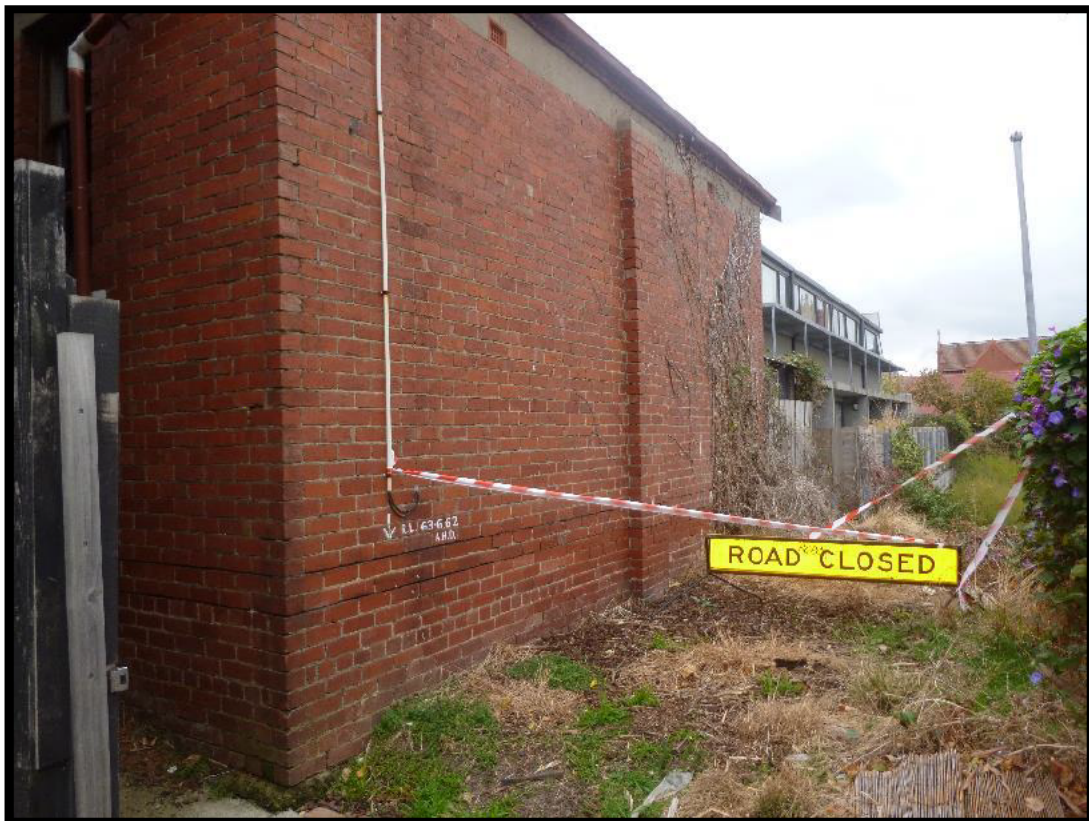
Photograph 18 – Photograph captured 29 April 2019. No evidence of movement and / or damage to the brickwork wall along the south boundary of 42 James Street, at the top of the battered ground to the subject land.
