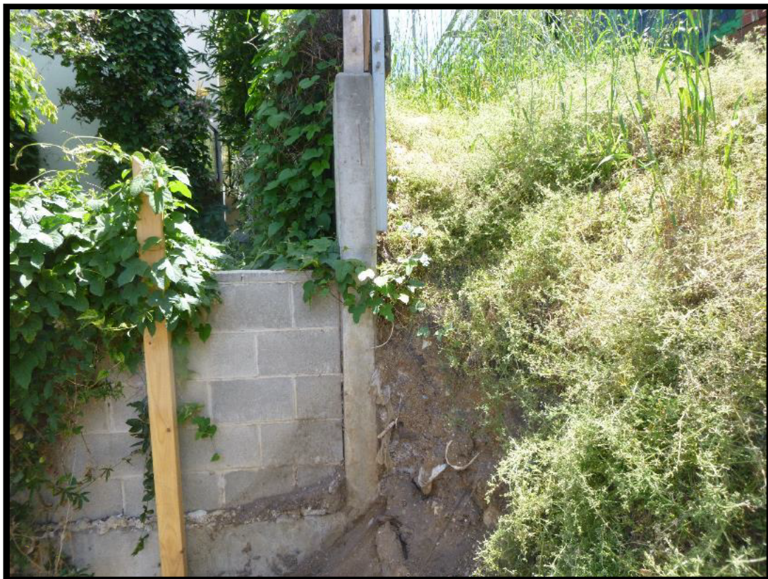
Photograph 8 – Photograph captured 19 November 2020. View of the western end of the subject land, looking west, at the north-east corner of 1 Campbell Grove (north-east corner of 1A Campbell Grove). Note vertical face of earth adjacent to concrete retaining wall.
