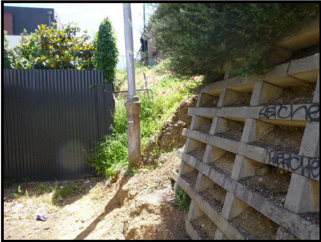
Photograph 3 – Photograph captured 19 November 2020. View of eastern end of subject land, looking west. Note spoil / loose material in laneway at the bottom of the batter. Slight erosion of material when compared to April 2019 (photograph 2).
