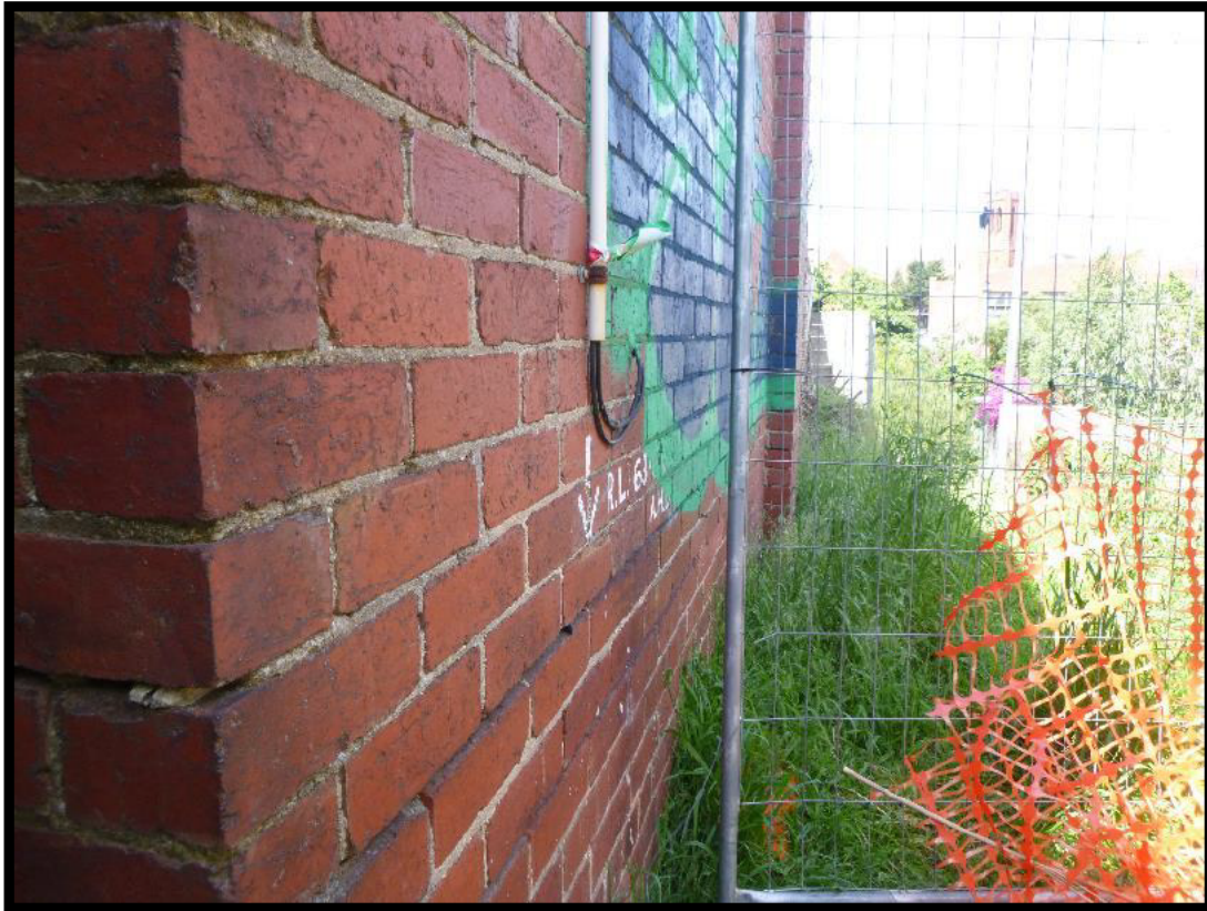
Photograph 19 – Photograph captured 19 November 2020. No evidence of movement and / or damage to the brickwork wall along the south boundary of 42 James Street, at the top of the battered ground to the subject land.
