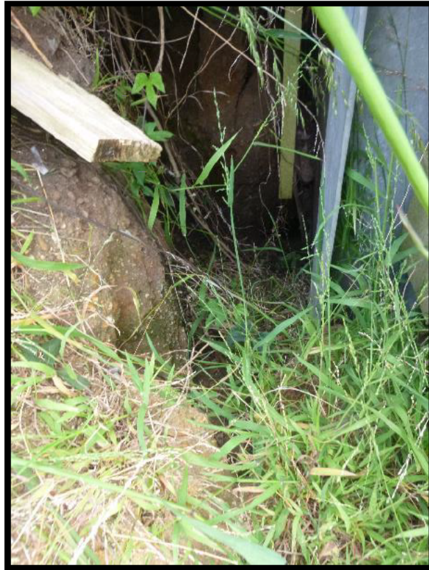
Photograph 21 – Photograph captured 13 October 2021. View of localised void beneath the south-east corner of the property boundary to 42 James Street, with the void appearing to extend beneath the south-west corner of property to the east of 42 James Street.
