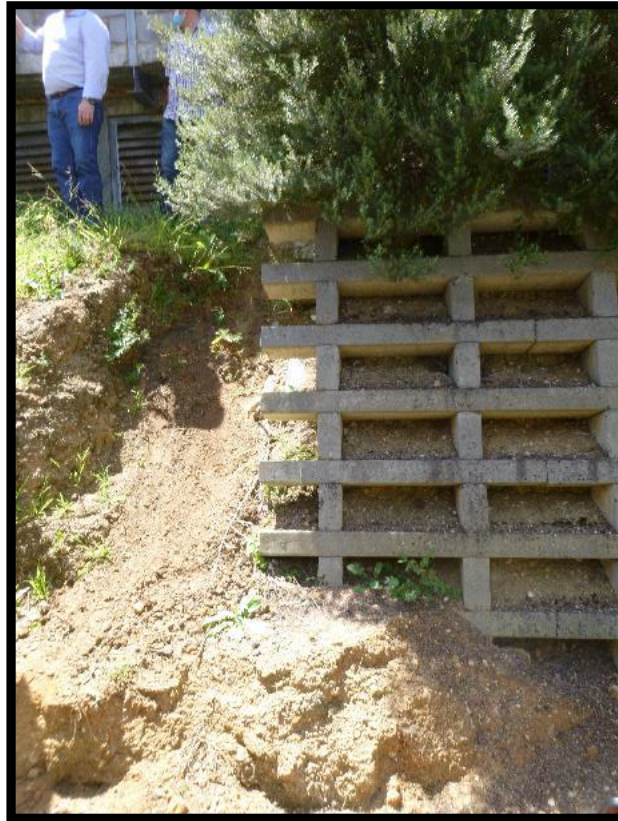
Photograph 5 – Photograph captured 19 November 2020. View of the eastern end of the subject land, looking north. Note localised erosion of land resulting in steep slope adjacent to crib wall.
