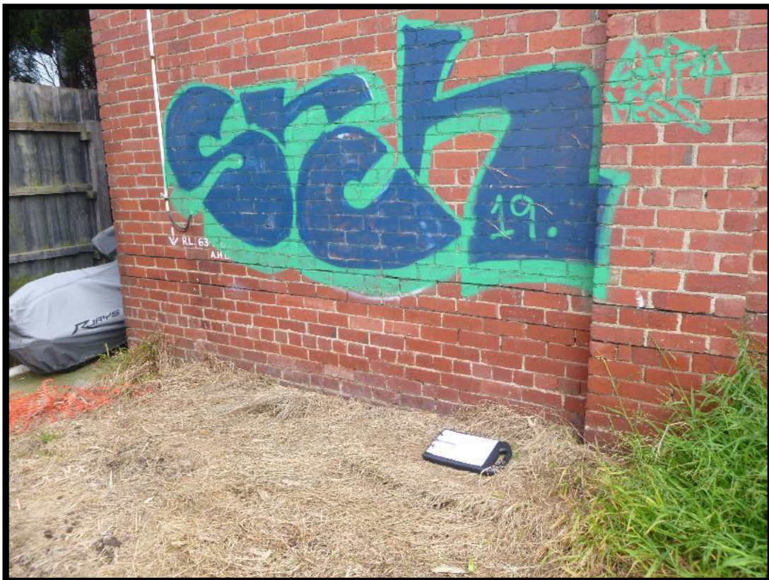
Photograph 20 – Photograph captured 13 October 2021. No evidence of movement and / or damage to the brickwork wall along the south boundary of 42 James Street, at the top of the battered ground to the subject land.
