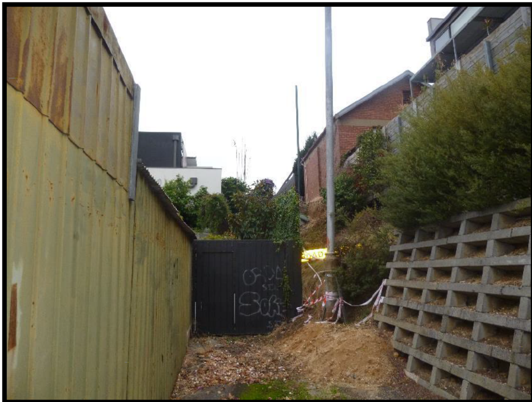
Photograph 2 – Photograph captured 29 April 2019. View of eastern end of subject land, looking west. Note spoil / loose material in laneway at the bottom of the batter.
