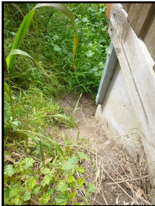
Photograph 12 – Photograph captured 13 October 2021. View of the western end of the subject land, looking east, at the north-east corner of 1 Campbell Grove (north-east corner of 1A Campbell Grove). Erosion of ground adjacent to retaining wall evident compared to November 2020 (photographs 7 – 9).
